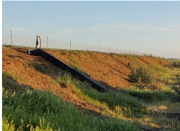
Photograph 3 – Pond Desludging Infrastructure
